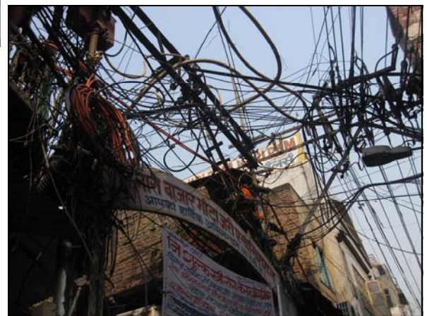
Old Delhi: This photo shows that electrical codes are not as strict as they are in the United States, which can pose health hazards to the public.
